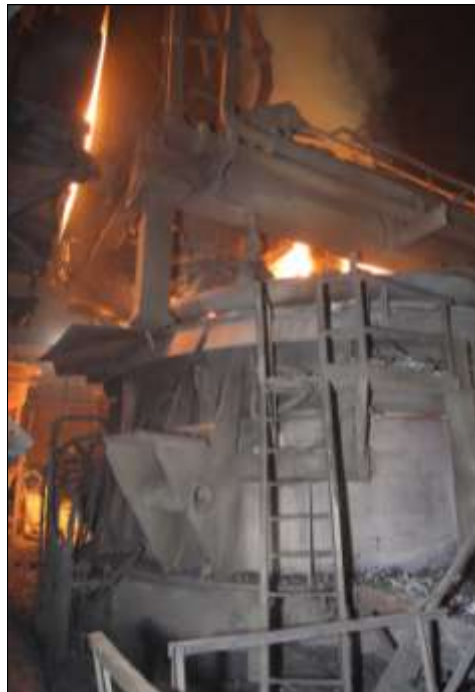
The electric arc furnace, used to melt iron and steel at the facility.
