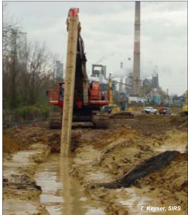
Construction of the 70-foot deep barrier wall in 2007 for the groundwater remedy at the site.
