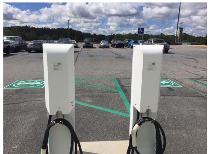
Level 2 Electric Vehicle Charging Stations at the Cape May-Lewes Ferry Terminal
