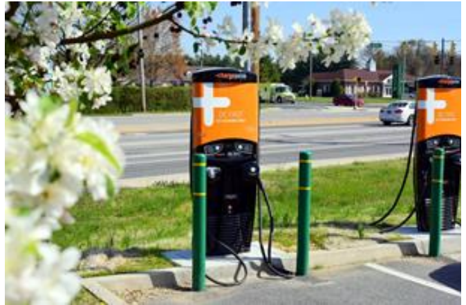
DC Fast Charging Stations at Royal Farms in Dover
