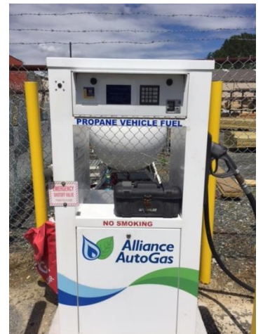
Propane Fueling Station in Rehoboth Beach
