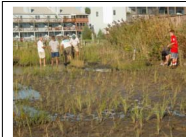
Boy Scouts install the few remaining plugs of Spartina alterniflora in disturbed tidal wetland.
