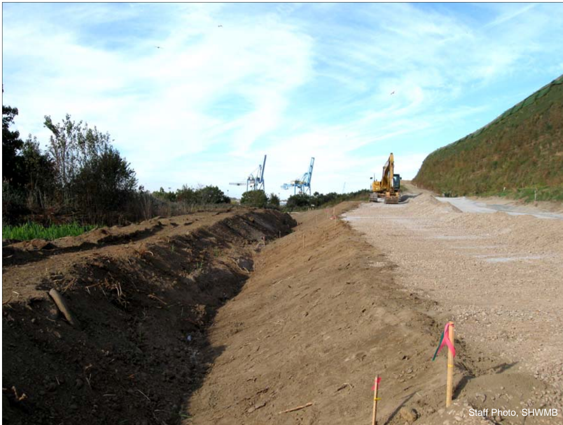
A track hoe is used to complete the earth-moving work on the lower tier of the Mechanically Stabilized Earth berm. The Port of Wilmington is located across the river from the landfill.
